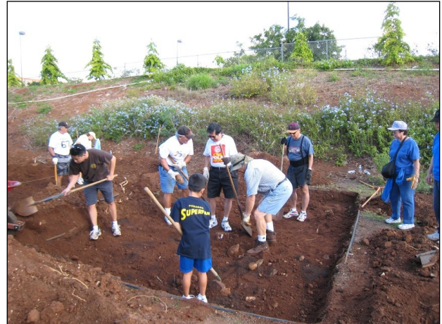
11/17/10 Volunteers from the Pearlridge Rotary helped to dig initial rose beds and amended the soil.
