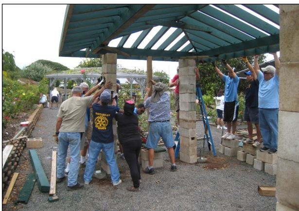
4/29/17 Members of the Pearlridge Rotary Club returned to help erect the center pergola and build planter boxes alongside the pergola.
